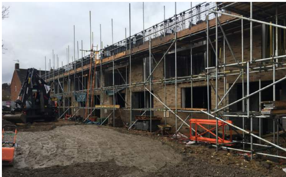
Construction of four, four-bed affordable homes at Chenduit Way, one of our infill sites
